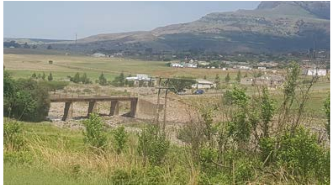
Mahai Bridge down!
